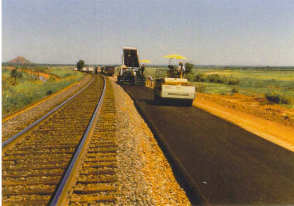
FIGURE 2a. Placing an HMA Underlayment on Subgrade during the Construction of a Second Track Next to an Existing Ballast Track.
