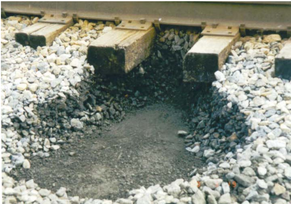
Figure 2b. Exposed HMA Underlayment in Trackbed with Ballast and Wood Tie Track
