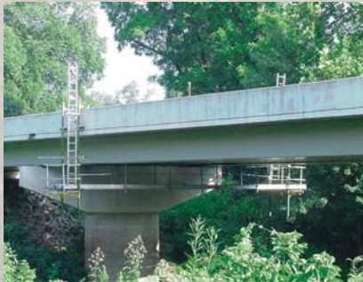
Scaffolding was put in place so that repairs to a Carter County bridge could be monitored monthly.
